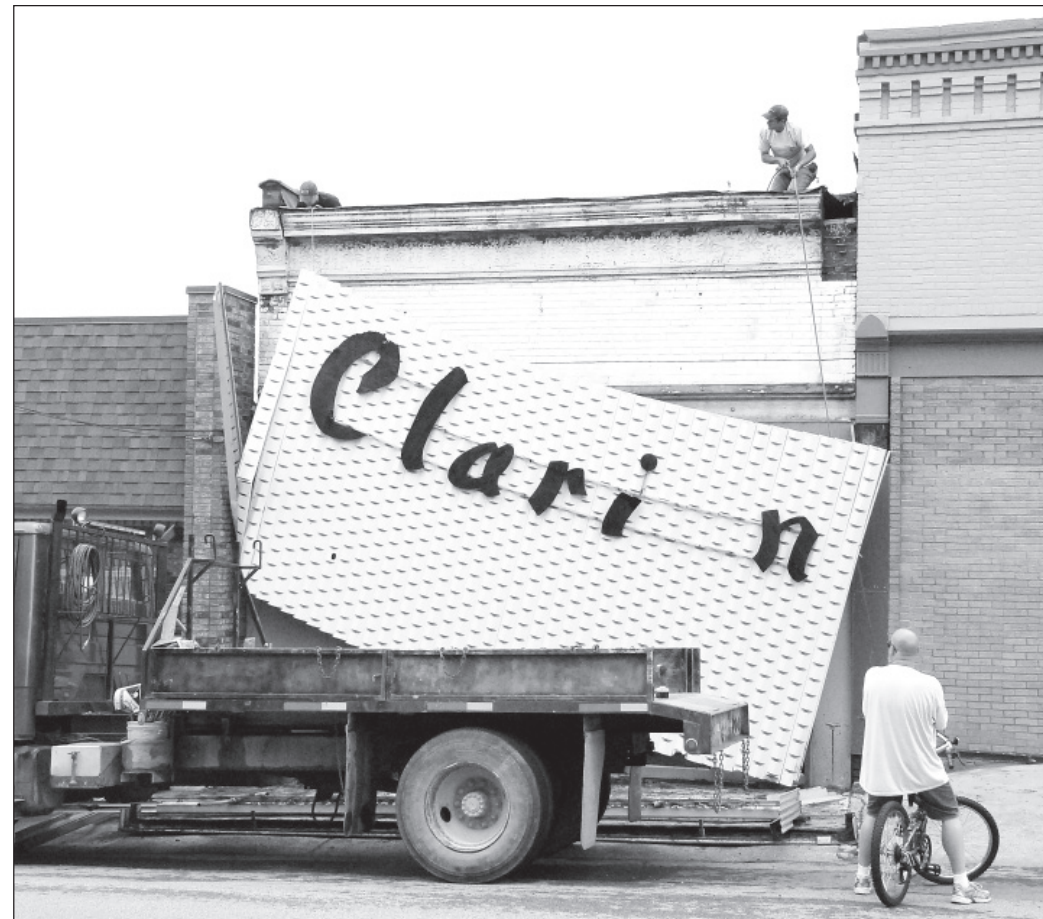
The historic "Clarion" sign was brought down last week as the office building receives revamping after 40 plus years.
